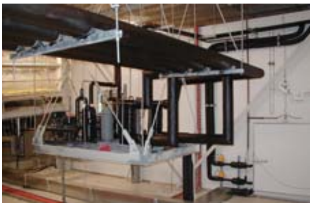
Fig. 2. R744 (CO 2 ) Condensing Unit installed in ceiling cavity
