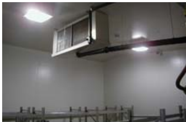
Fig. 3. Finned air cooler suitable for R744 (CO 2 ) refrigerant and installed in the cold store
